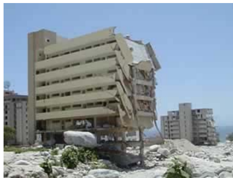
*Apartment in Caraballeda extensively damaged by passage of debris-flow front at least 3.5 m in height, leaving boulders (> 1m) on second floor of structure.* Source: http://pubs.usgs.gov/of/2001/ofr-01-0144/Venezuela/image033.jpg , accessed May 18, 2006.
